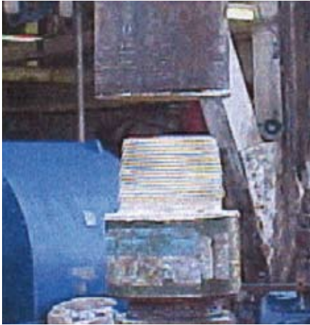
Figure 7 Dope condition of top drive saver sub & main shaft
